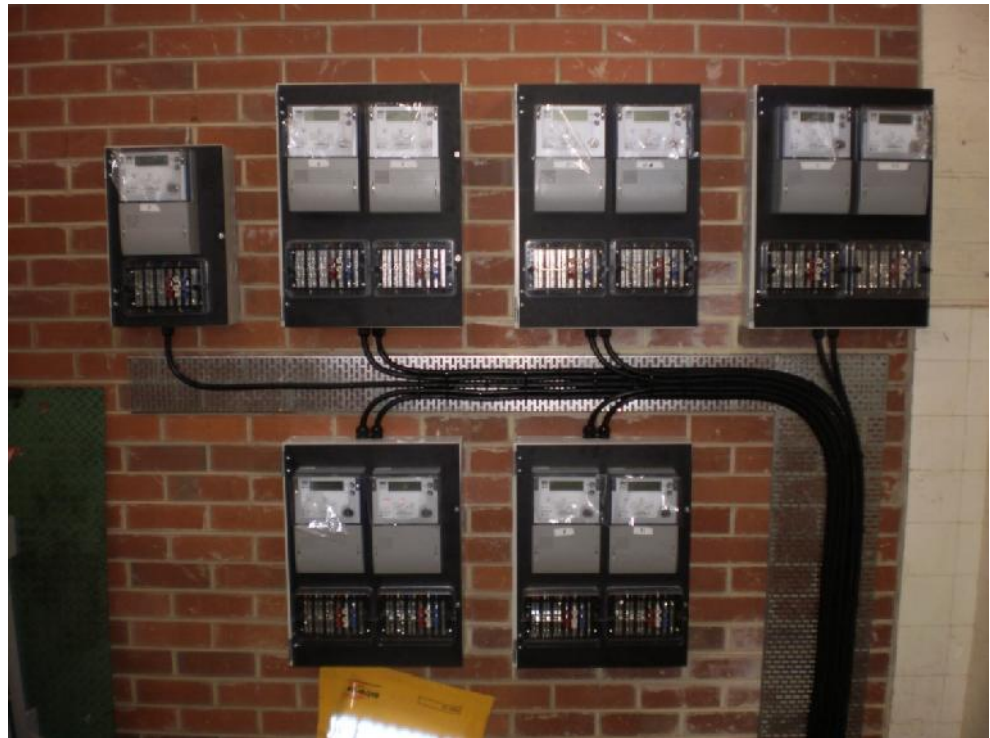
Multiple smart meter installation
