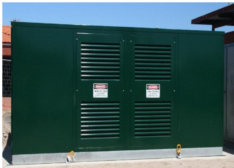
11kV\415VAC Kiosk with RMU & LV Switchgear
